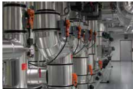
Heating/cooling control centre
