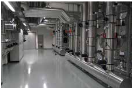
Heating/cooling control centre
