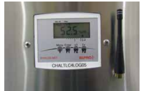
Temperature and humidity measurement with wireless link
